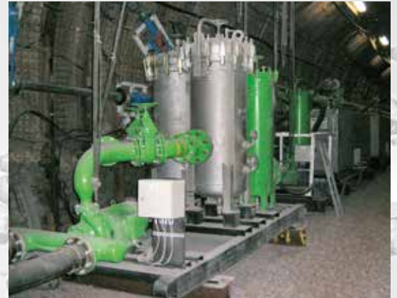
Stationary pump station for HFA supply
