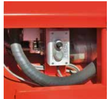
Filling pump for circulation pumping of hydraulic oil
