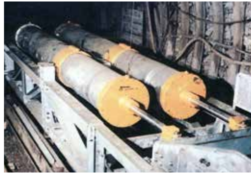
Cylinders for pneumatic belt tension
