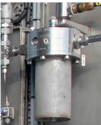
Filter with Hazardous area clogging indicator VDHA with 316 stainless steel junction box (indicator approved with ATEX and IECEx; CSA/UL) on a Wellhead Control Panel.
